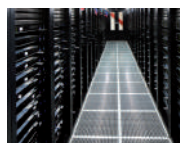
Telecom base station
