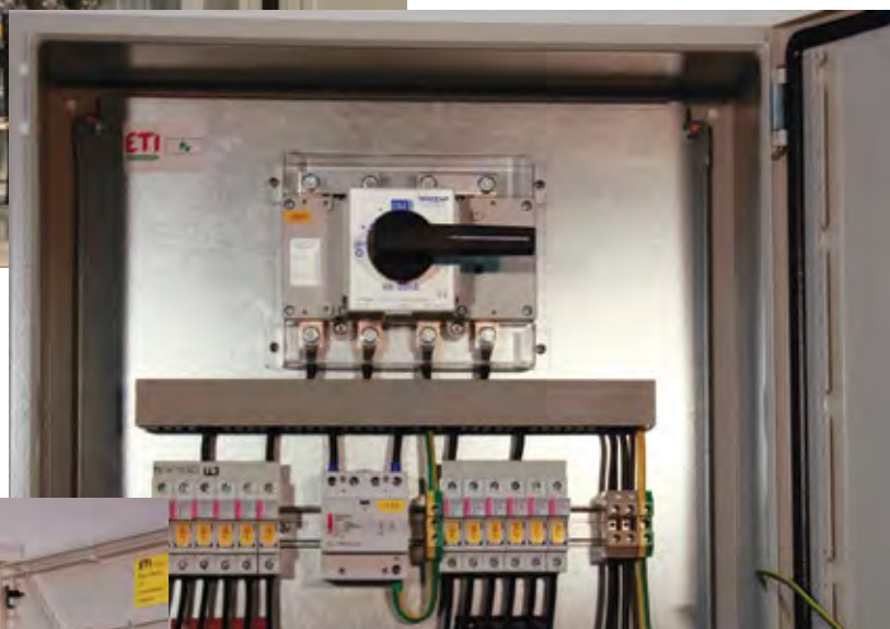
DC junction box (CH gPV fuses)
