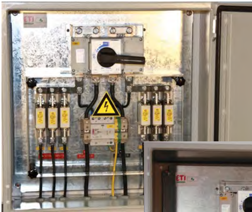
DC junction box (NH gPV fuses)
