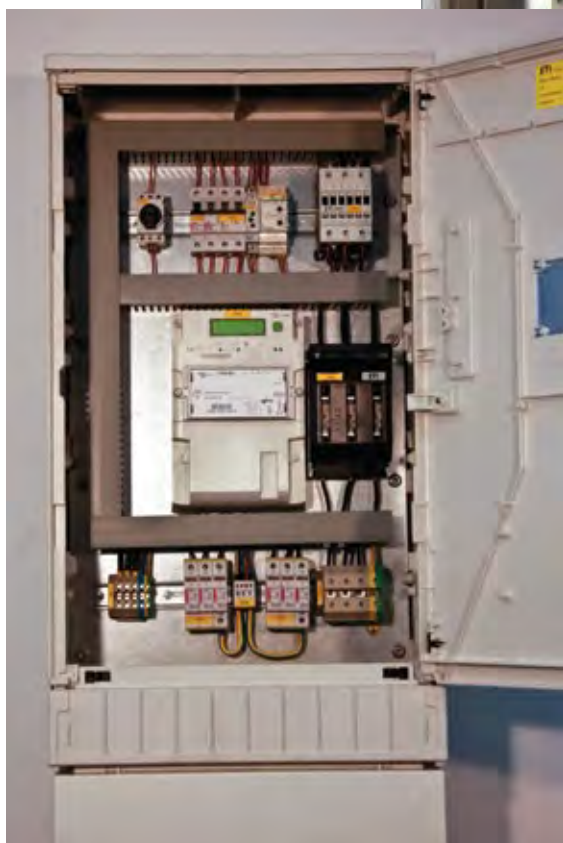
Meter distribution cabinet
